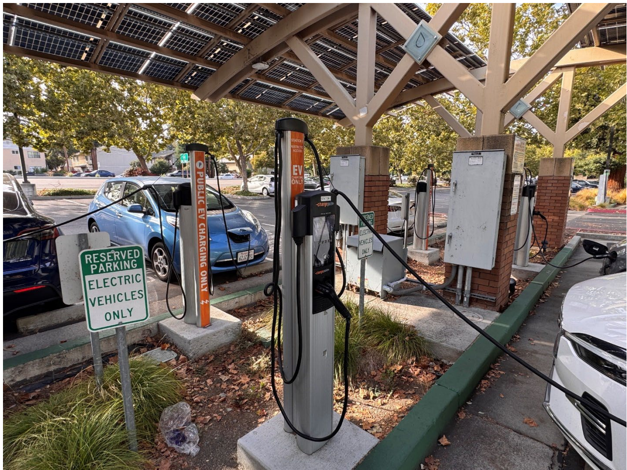
Figure 2-9. Existing Staff and Public Level 2 EV Charger
