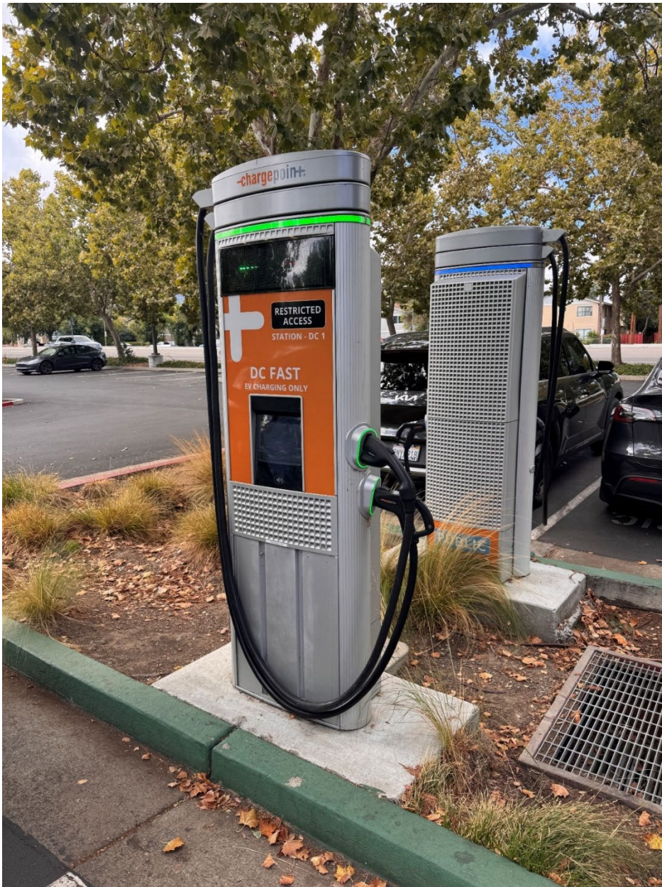
Figure 2-11. Existing Level 3 EV Charger
