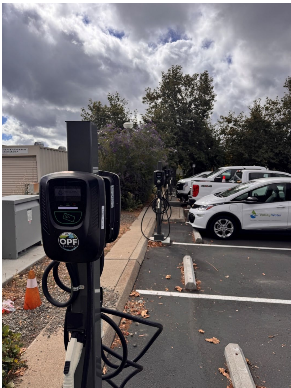
Figure 2-10. Existing Fleet Level 2 EV Charger
